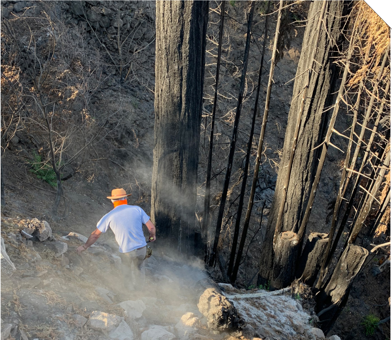
Previous Page and Above: Property clearing and rebuilding process off Braemoor Drive. Photos by Trevor Jones
